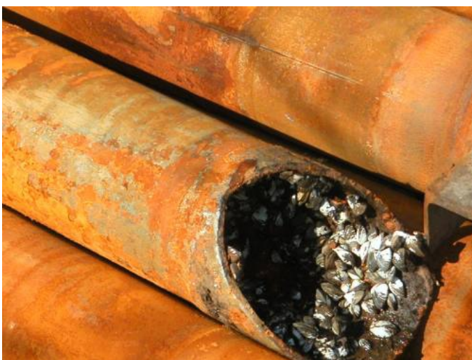
At Lake Ontario in Canada, zebra mussels cling to the inside of a rusty pipe.
